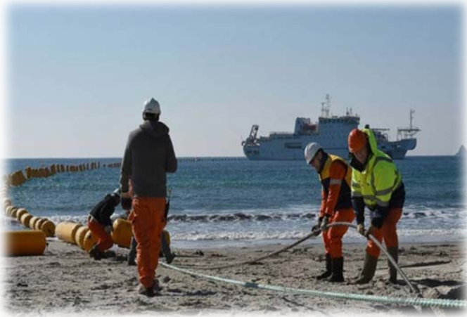
Submarine Cable Project
