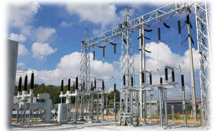
Power Substation Project
